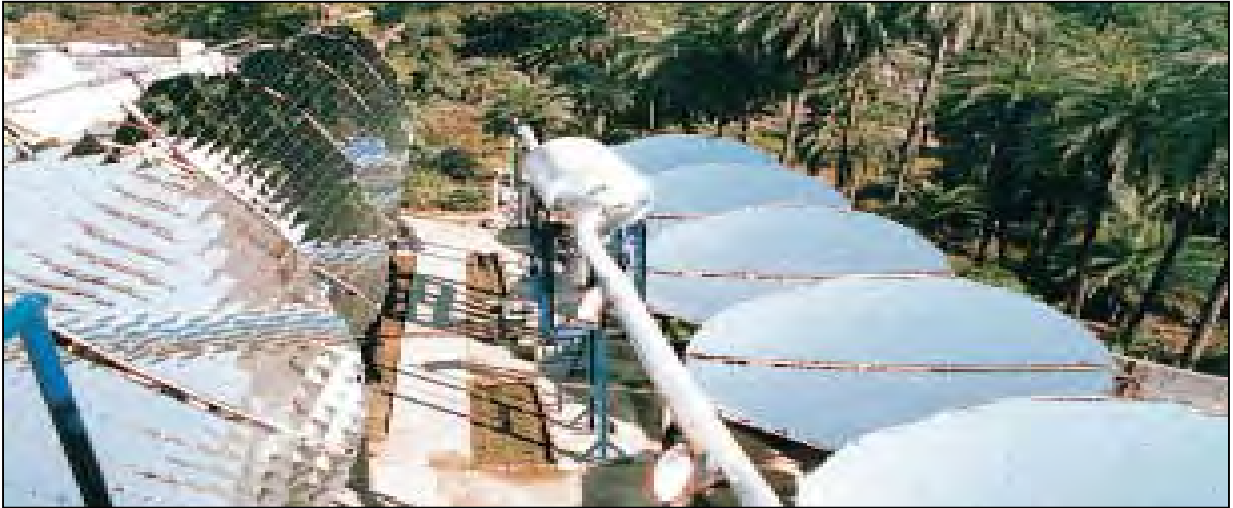
Figure 15: A Solar Energy System at Global Hospital, Mount Abu
